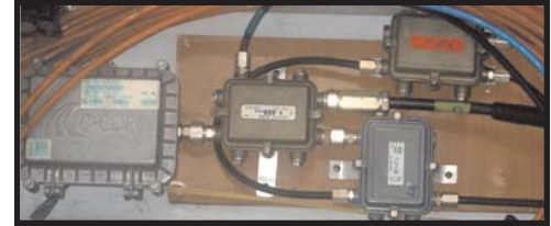
Node box inside
