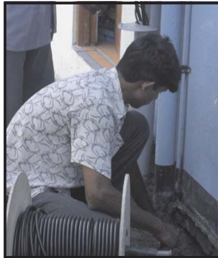
Drop Cable to home
